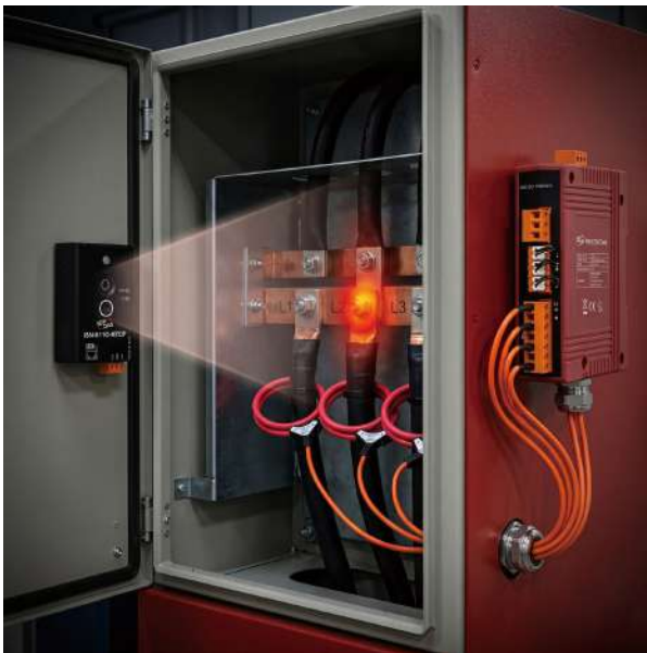
▲ Figure 3 | HV Switchgear Hotspot Monitoring Thermal imaging instantly detects switchgear hotspots, preventing electrical fires and downtime.
