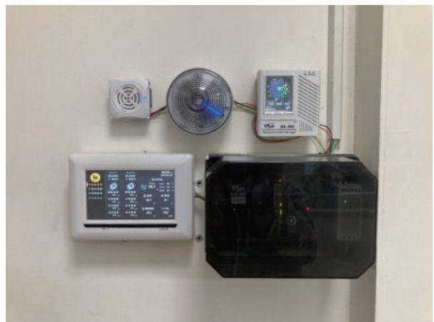
▲ Integrated monitoring system with TPD and on-site alarms.
