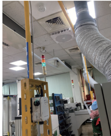
▲ Aluminum rails and straps are used to secure the nitrogen pressurized lines next to the two soldering machines.
