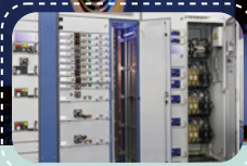
Main Electrical Box
